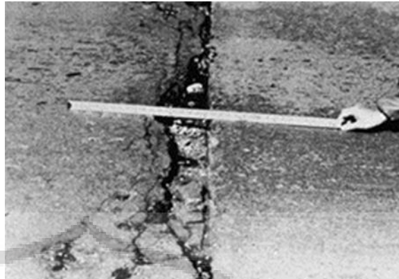
Gambar 2. 4 Kerusakan Spalling Joint
