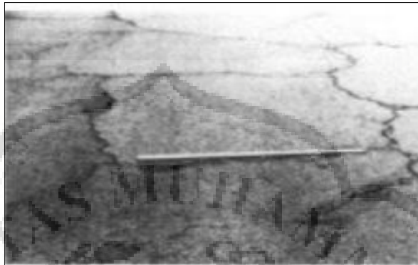
Gambar 2.9 Retak blok ( Block Cracking ) Sumber : Bina marga no.03/MN/B/1983
