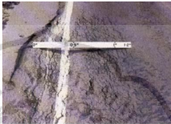
Gambar 2.3 Sungkur ( Shoving ) Sumber : Bina marga no.03/MN/B/1983
