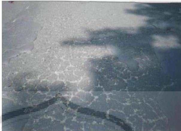
Gambar 2.11 Pelepasan Butir ( Weathering/Raveling ) Sumber : Bina marga no.03/MN/B/1983
