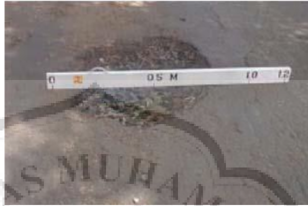
Gambar 2.14 Lubang ( Pothole ) Sumber : Bina marga no.03/MN/B/1983
