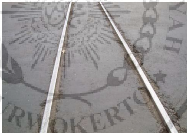
Gambar 2.16 Rusak Perpotongan Rel ( Railroad Crossing ) Sumber : Bina marga no.03/MN/B/1983
