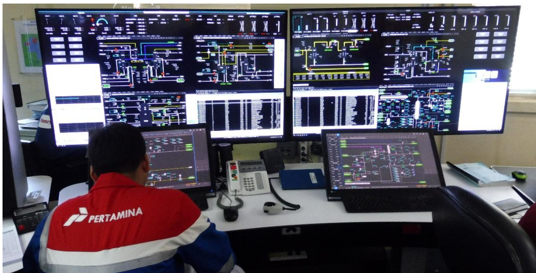
Gambar 2.8 HMI DCS Honeywell Orion Console
